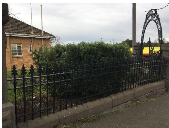
Figure 3.72 Ninth section of Barkly Street fencing. Some lifting and staining of bluestone base.
