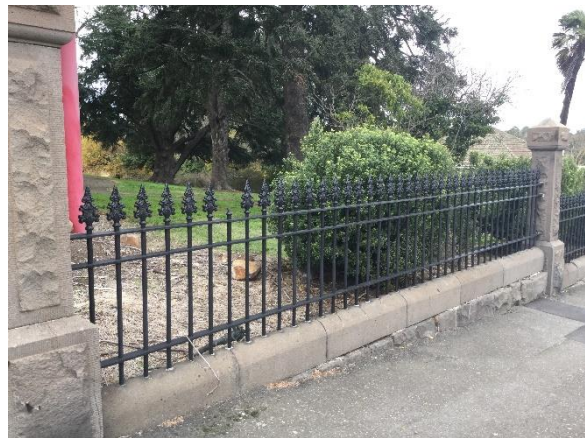
Figure 3.66 Third section of Barkly Street fencing. Some cracking to foundation top. One arrowhead of palisade lost.
