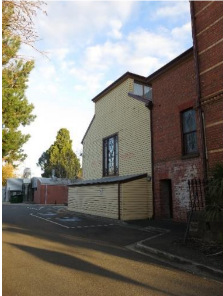
Figure 3.11 View of hall to the rear of former Free Library from driveway to east. Between the hall and the original Free Library fronting Barkly Street is the utilitarian red brick façade of the eastern end of the link. Damage to bricks to the lower section of this wall indicates that an earlier addition has been removed. The east elevation of the hall has weatherboard cladding extensively replaced at the time of the 1998–2000 alterations and additions to the (then) former Ballarat Secondary College. The single-storey store attached to the hall was also added as part of these works. (May 2020)
