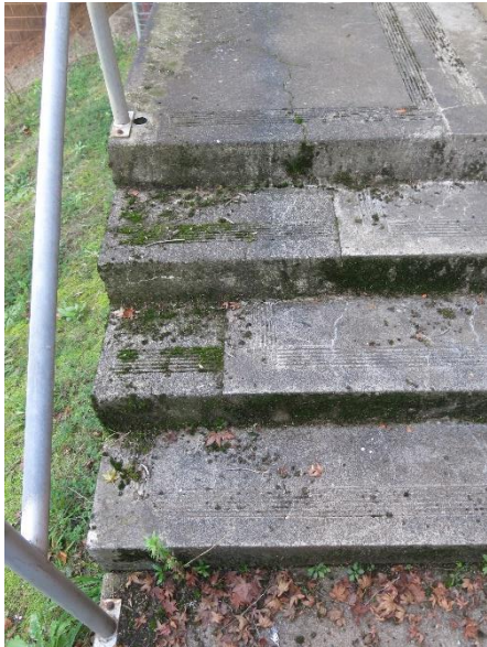
Figure 3.32 Altered concrete stairs to north entry of west elevations of former Ballarat Girls High School. (May 2020)
