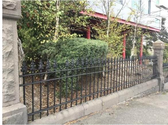
Figure 3.64 First section of Barkly Street fencing. Two arrowheads of palisade are lost.
