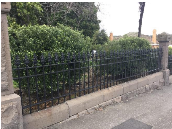
Figure 3.67 Fourth section of Barkly Street fencing. Some lifting of bluestone base. One arrowhead of palisade is lost.
