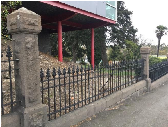
Figure 3.65 Second section of Barkly Street fencing, small chips to edges at joints.
