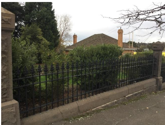
Figure 3.69 Sixth section of Barkly Street fencing. Fine cracking to nearest base stone. One arrowhead of palisade lost.
