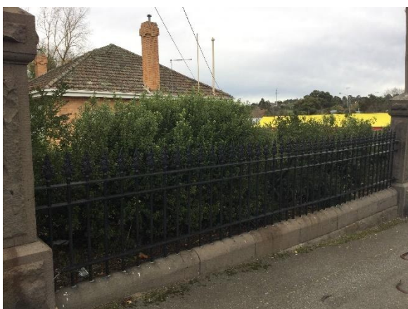
Figure 3.71 Eighth section of Barkly Street fencing. Some bird droppings and some staining from rusted palisade bases.
